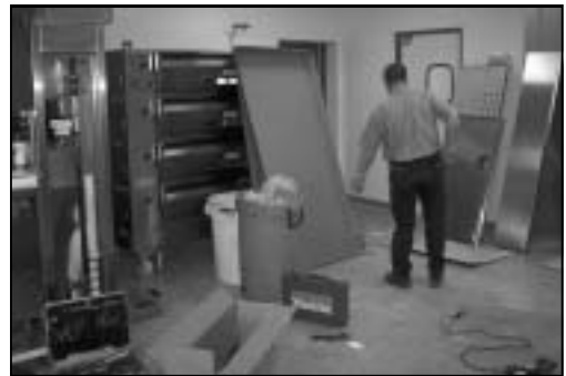
A worker readies Pierce's new bakery. Many new changes and fresh updates are in the works at Pierce's Marketplace for mid-2008.
